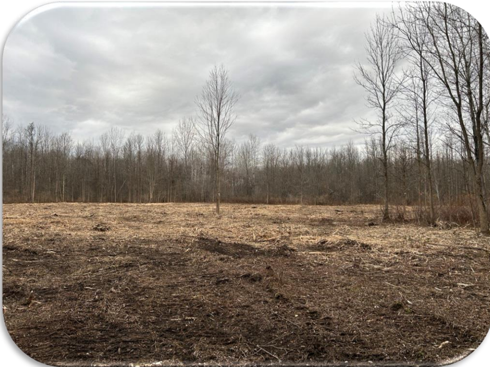
Cleared area for wetland pond Two Creeks Forest Conservation Area South Dundas
