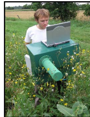
SNC staff maintaining telemetry unit and datalogger on a PGMN well.
