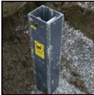
Figure 3: Tile drain control structure installed on a tile header for the WEBS – controlled drainage BMP.
